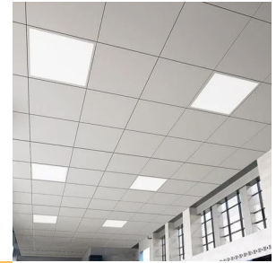
Grid ceiling (lay-in tiles, service access)
